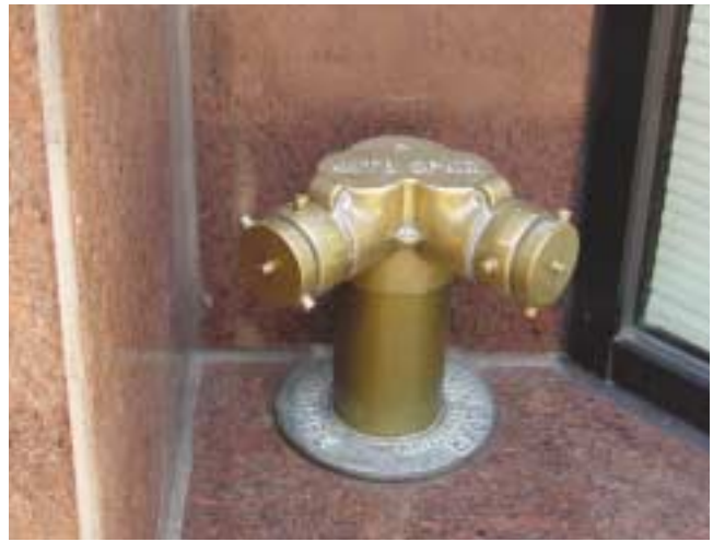
(Fig. 5.6) This FDC is mounted too close to a wall. Other obstructions could be fences, pipes, downspouts, vegetation, etc.
