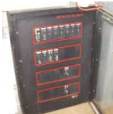
(Fig. 6.1b) Control panel.
