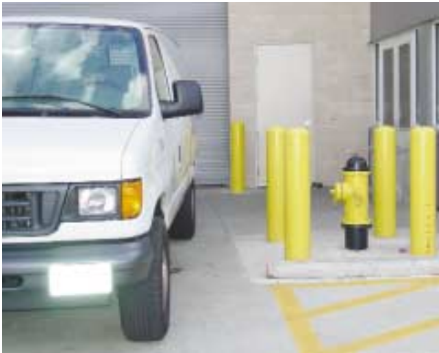
(Fig. 2.14) This hydrant should not have been located where it is likely to be blocked. Loading docks, by nature, will likely have vehicles parked. This is an example of building a potential deficiency into a facility. The truck could prevent use of the large pumper connection or cause the base to be kinked when used. Note the yellow bollards which protect the hydrant from vehicle collision.
