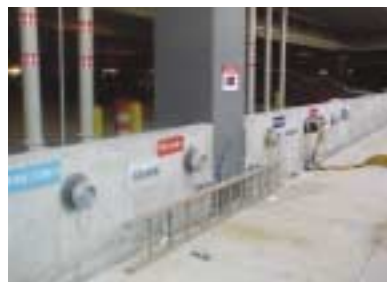
(Fig. 4.13) FDCs for separate manual dry standpipe systems in a large parking garage.
