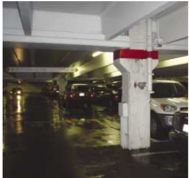
(Fig. 4.6) Stripe on column to identify hose connection location in a parking garage.
