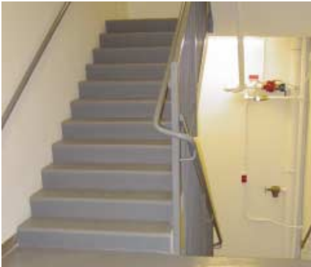
(Fig. 4.2) Hose connection on intermediate landing as viewed from the main landing where the stair entry door is located.
