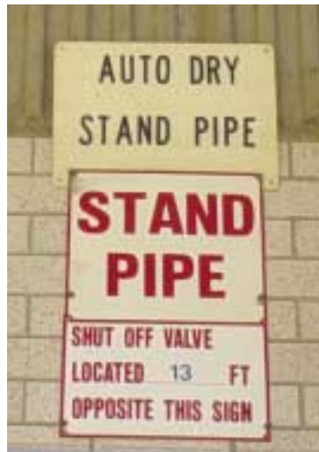
(Fig. 3.3) Exterior sign showing valve location (in this case for a standpipe system).
