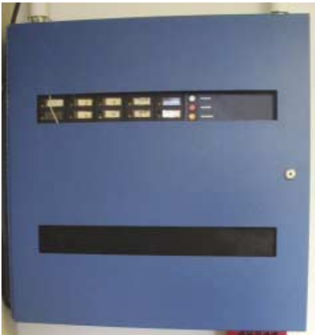
(Fig. 6.2) Simple fire alarm control panel with lamps and zone labels for annunciation.
