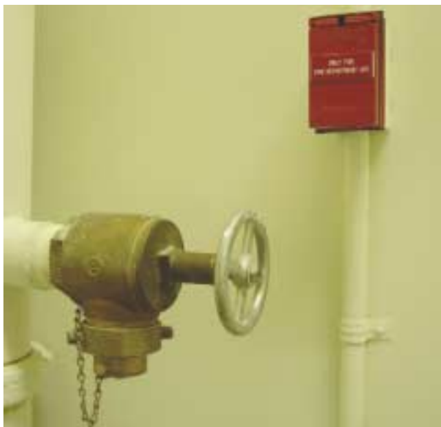
(Fig. 7.1) Firefighter emergency power receptacle next to a standpipe fire hose connection inside of a stair enclosure.
