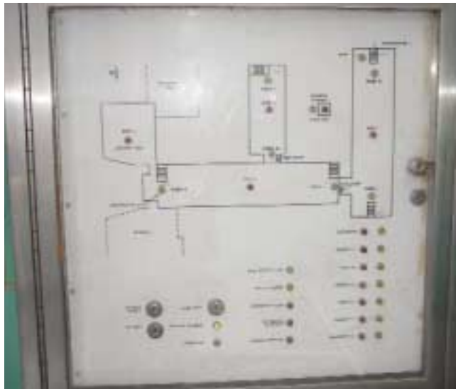
(Fig. 6.5) One of two annunciators in a building with four wings, which fronts on three different streets.
