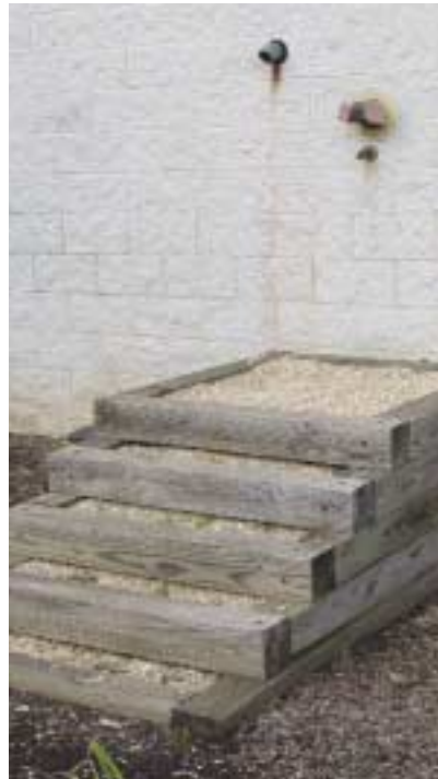
(Fig. 5.10) A platform built up to reach an FDC creates a hazardous condition. This should not be considered as equivalent to positioning the FDC at a proper height above grade level.
