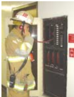
(Fig. 6.8a) Fire officer speaking into the handset at the control panel for a fire department communication system. This panel also houses the handsets used by firefighters at remote jacks.
