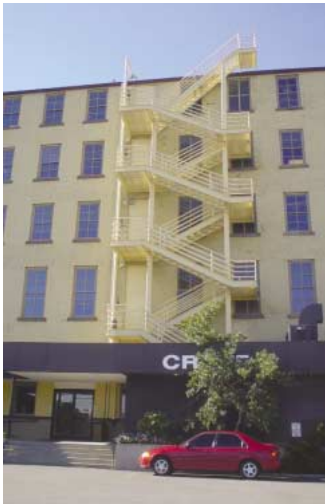
(Fig. 4.1) A dry standpipe in an exterior stair. The FDC inlet is to the right of the building entrance, the riser pipe extends through the left side stair landings, and hose connections are at each level, including the roof.
